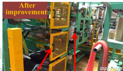
Description : safety net and emergency stop
